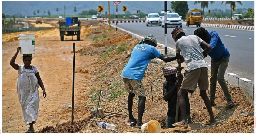
Govindan and other workers, including a woman, digging a pit for an electricity pole near the Seed Access Road in Anaravali. (Devika Hussaini, along with other workers, returning home after a strenuous day's work near Venkayyapalem in Thullur taluk of Cuddalore district in May 2024)
