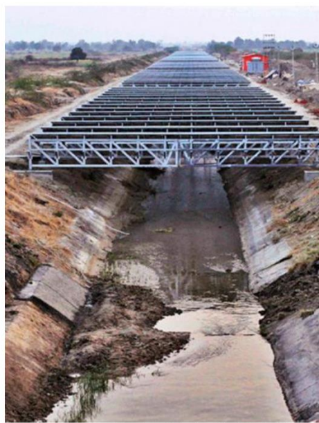
Solar panels seen installed above the Narmada canal in Chandrasan village, Gujarat, in 2012. The State hosted India's first canal-top photovoltaics. AP
